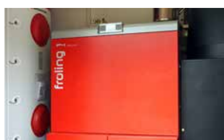
The two Froling pellet boilers are reliable and robust.
