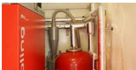
The pipework in the plant room has been fully insulated.
