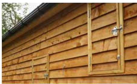
Fuel store inspection hatches and fuel filling nozzles have wooden doors.
